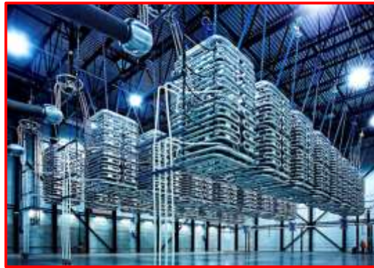
Substation of a UHVDC Line
